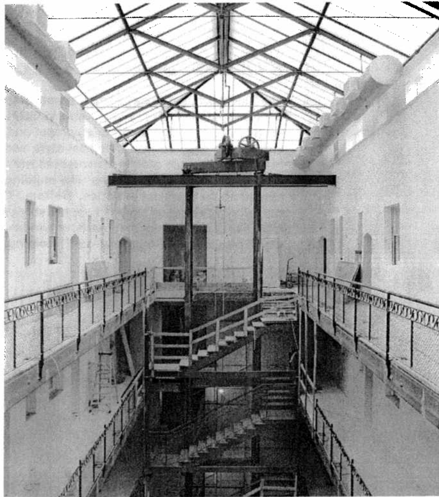
Individual units in the Yale Apartments open onto the atrium, which is topped by a glass-and-metal skylight.
